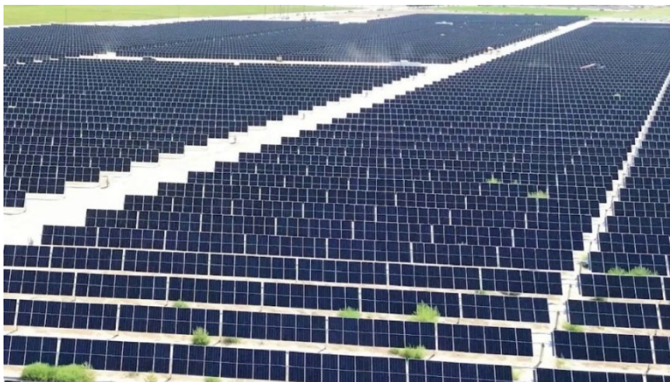
Fig. 5. EPE Facility in San Elizario, TX (about 60 miles SE of Las Cruces, NM). Note the Russian thistle beginning to grow to at least half the height of the PV modules.
